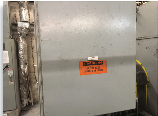
Figure 2 - The control chassis was typically mounted in a separate cabinet but closely coupled with the cabinet containing the rectifier bridge.
